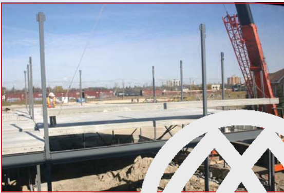
Construction on the northeast quadrant: top to bottom - pouring concrete grade beams; installing structural steel; installing concrete hollow core.
